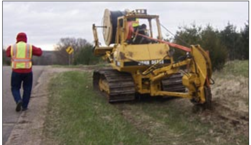
(above) A plow blade installs the main fiber optic cable line in the ground.
