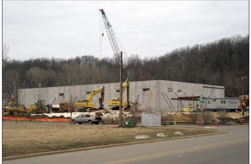
above: Subcontractors are setting prefabricated concrete wall panels into place for the Air Motion Systems headquarters at Whitetail Ridge Corporate Park (River Falls, WI)
