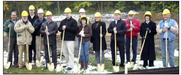
Community leaders joined Jeff and Kristi Cernohous (center of the photo) at a ceremonial groundbreaking to mark the start of construction on a 22,000 square foot addition to Interfacial Solutions' existing facility.
